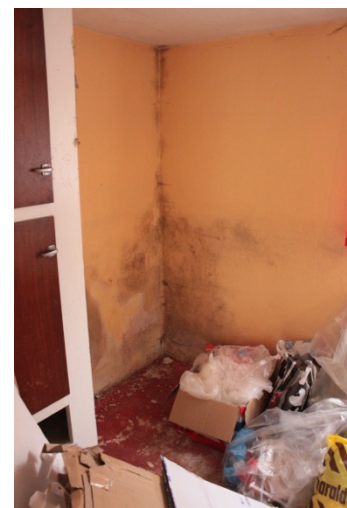
Mold and mildew in a tenant's basement. Photo: Judith Doyle
